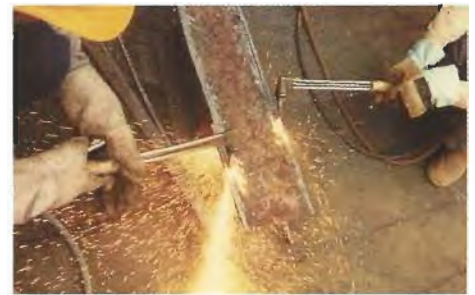
The beginning of a cut on a 6 foot (2 meter) long 1/2" (125 mm.) thick plate shows faster preheating and piercing using HGX Fuel Gas and oxygen versus L.P.G. and oxygen.
